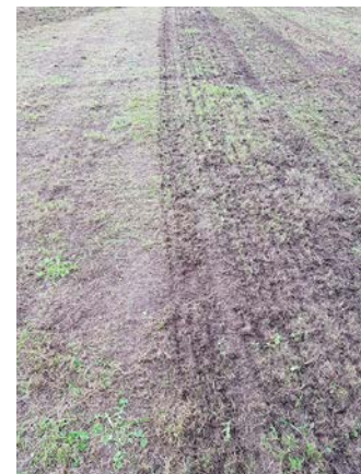
A plot in Devon being prepared for the establishment of wildflower seeds in early October. The ground has been cleared with a flail collector and the right-hand side has had one pass with a Scarrow.
